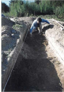
大地を掘り窯の胴体をつくる Dig a sloping trench up a hillside for the body of the kiln.
